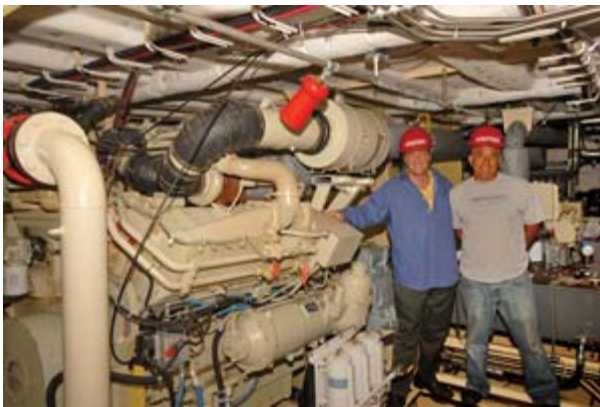
Two Circle Line executives with the Cummins KTA38M1 diesels: Robert Maher, CEO, (left) and Gus Markou, the company's director of marine operations.
